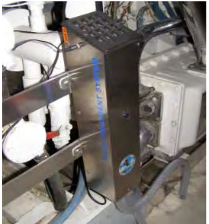
Holding Tank Ventilation System
